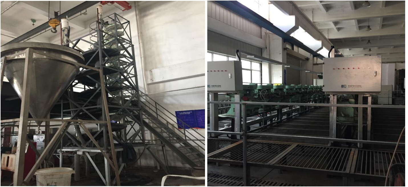
Figure 3: Hunan Research Facility spiral and flotation circuits
