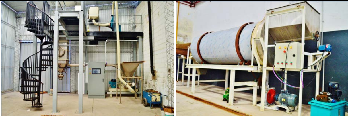
Figures 4-5: Rincon Lithium Project – Stage 1 industrial-scale pilot plant operations
