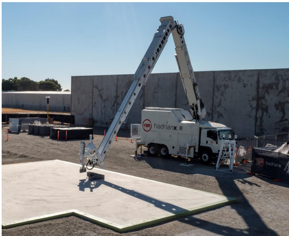
The building of an 'F' structure in progress. The two-course F structure comprises every block configuration and combination required for the build of a full home structure.
