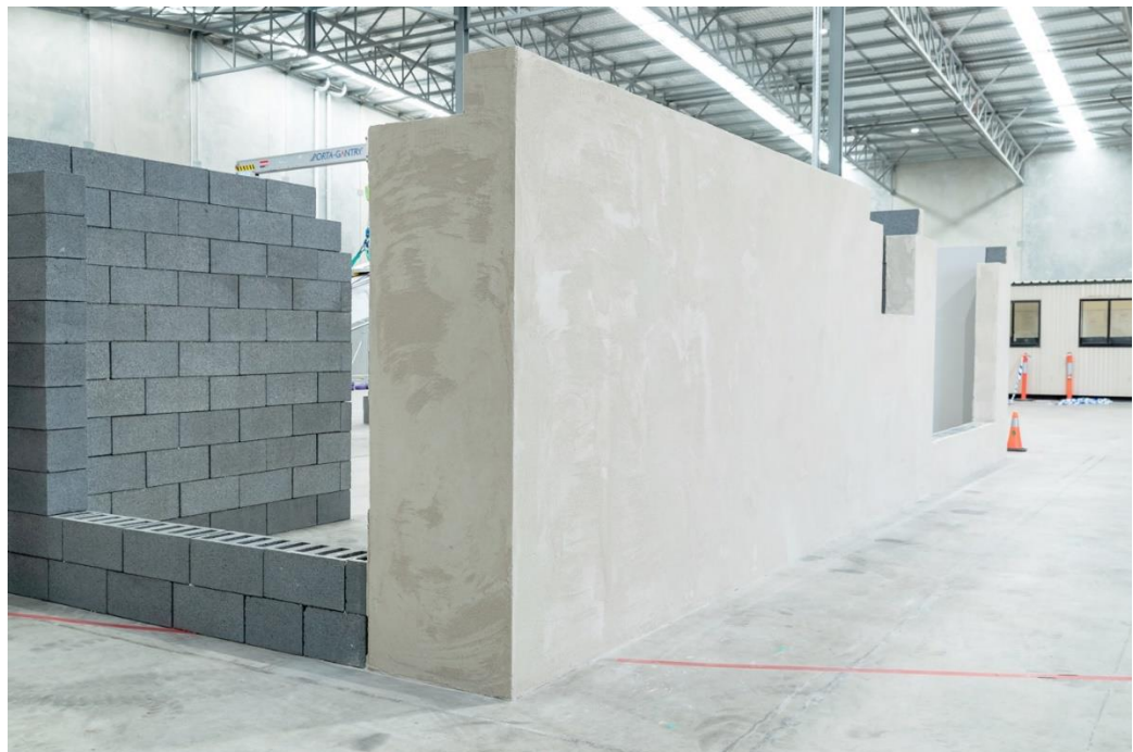
The finished three-bedroom, two-bathroom structure built at FBR's test facility with the Hadrian X in under three days
