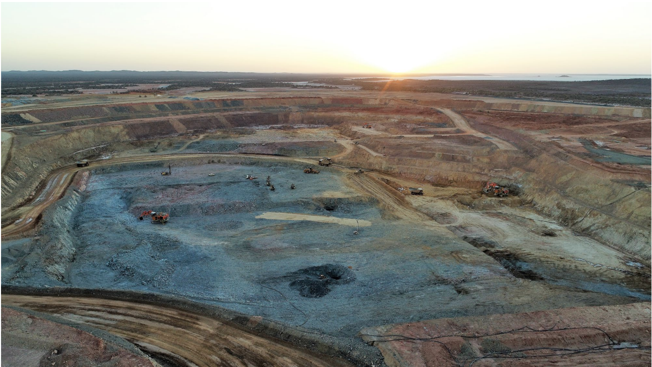
Figure 3: Photograph of mining activities at Heffernans, part of the Jupiter open pit. Note first mining at Heffernans occurred in December 2017 when the deposit was situated within a 25m high hill.
