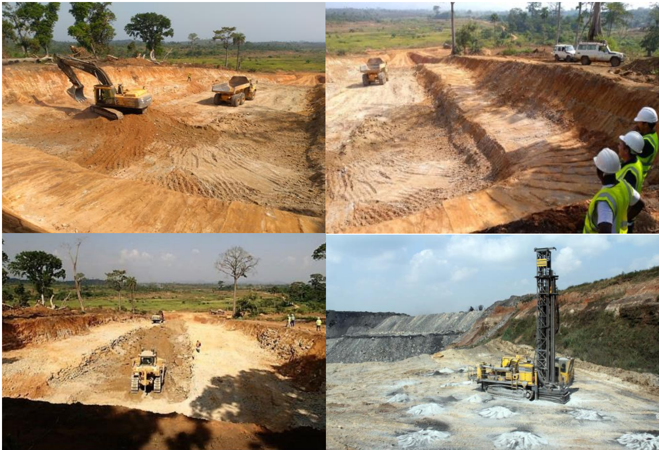
Figure 4: Tongo Boxcut preparation and excavation activities, including preparation for drilling and blasting for the Mine Portal
