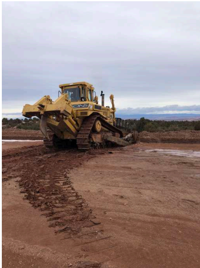
Photo 1: Ramping down off an existing oil well pad at Anson's Paradox Lithium Project.
