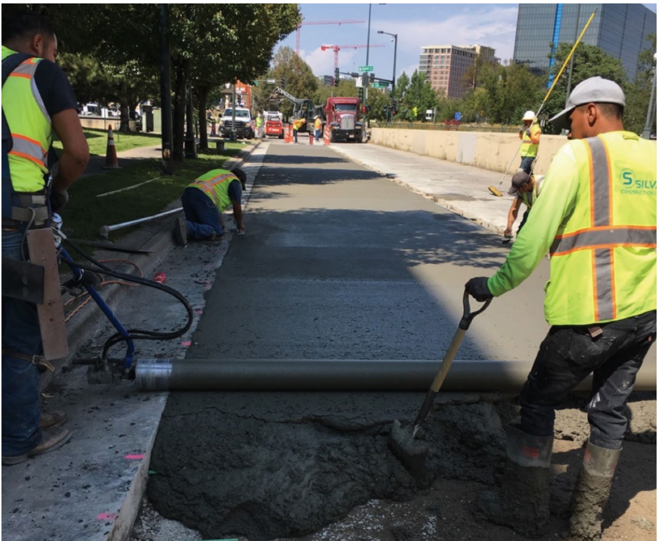
Figure 3 – One of Two New Trial Sections of Concrete Pavement in second trials
