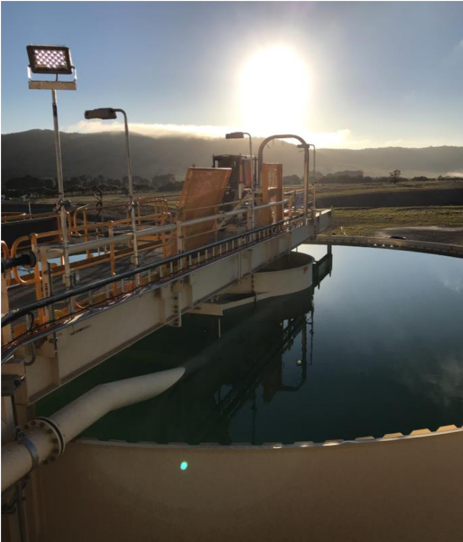
Figure 5 Tailings thickener undergoing wet commissioning.
