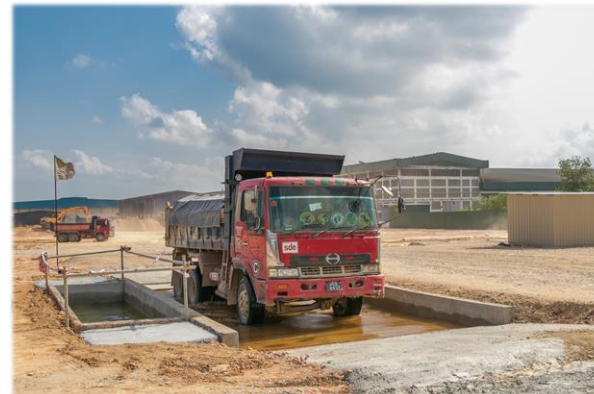
Vehicle wash down bay with sediment control
