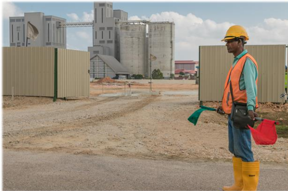
Site access control
