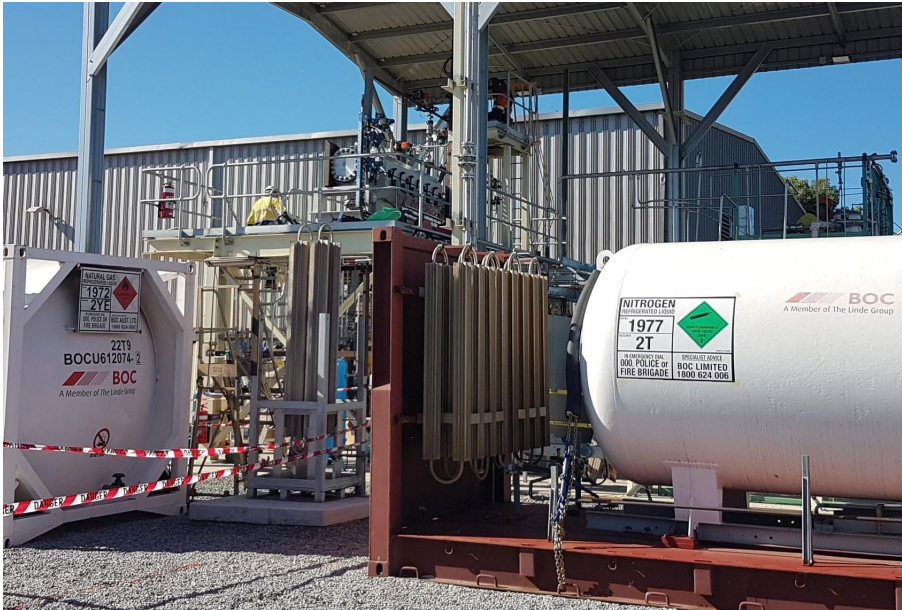
Photo 2 – MRL's new Reactor (top floor) at the Kwinana site, Western Australia.
