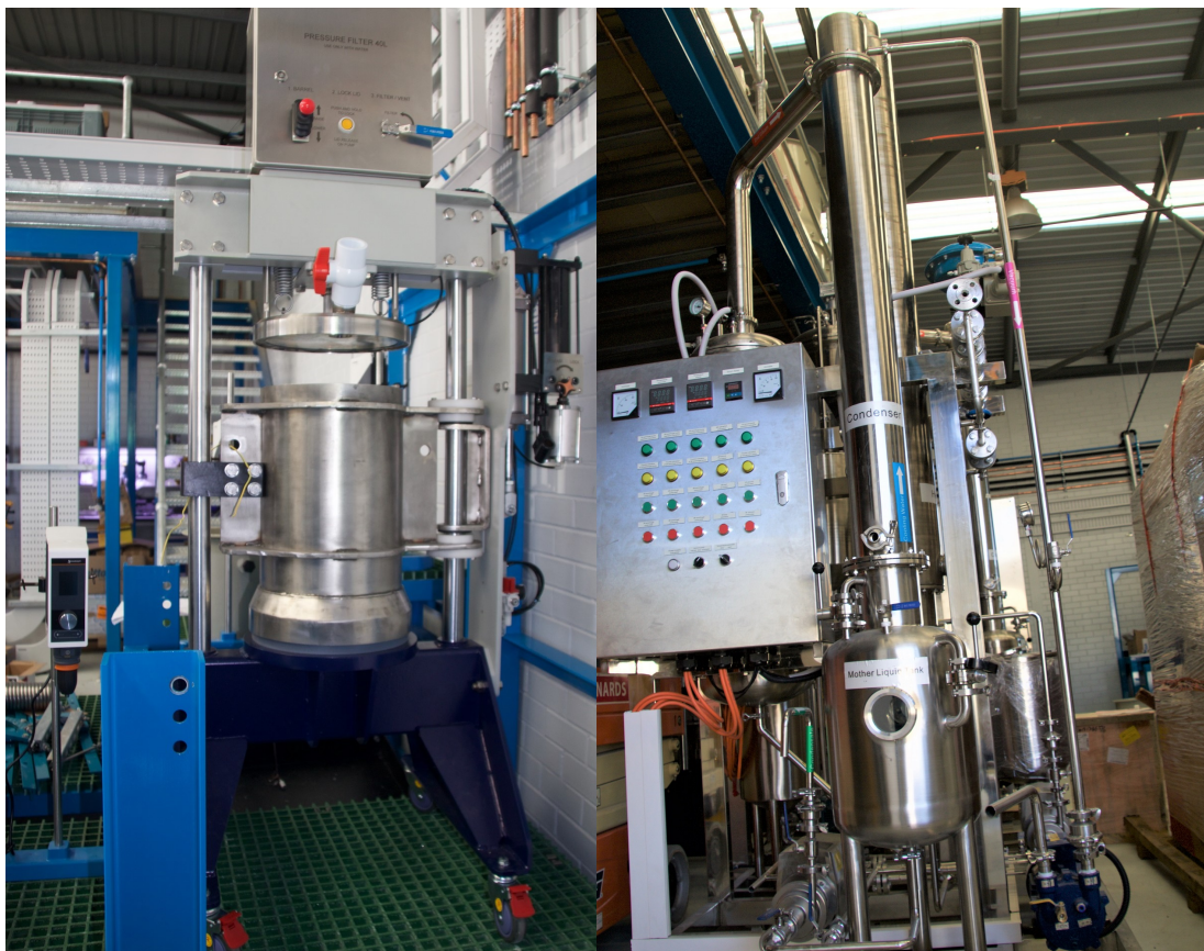
Figure 2a (left) & 2b (right). 2a Pressure filter and 2b crystalliser installed, awaiting plumbing.
