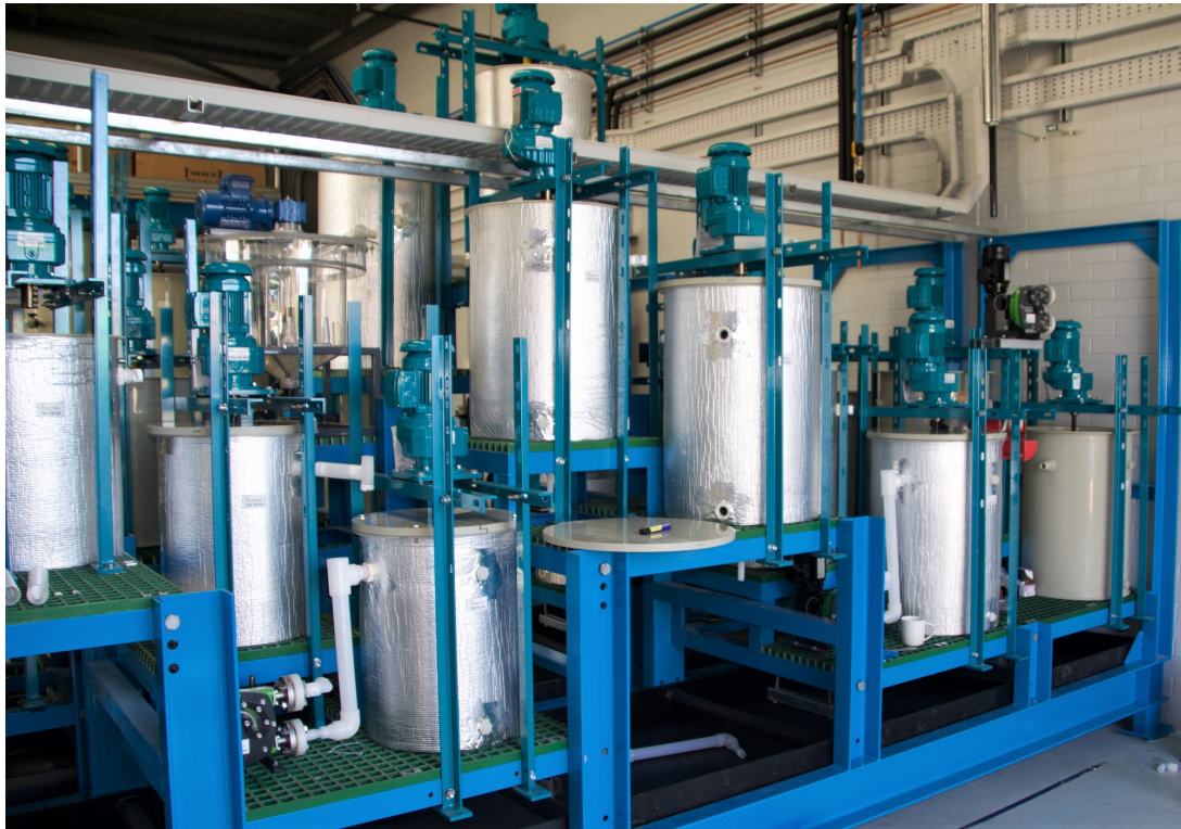
Figure 1. Pilot Plant leach circuit skid with leach reactors installed and fit-out in progress.
