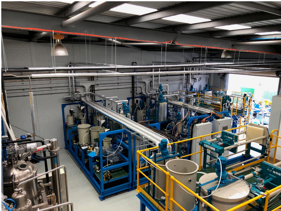
Figure 2. Pilot Plant on 12 April 2015 all major mechanical equipment installed, with electrical fit-out and piping well advanced for completion on 30 April.
