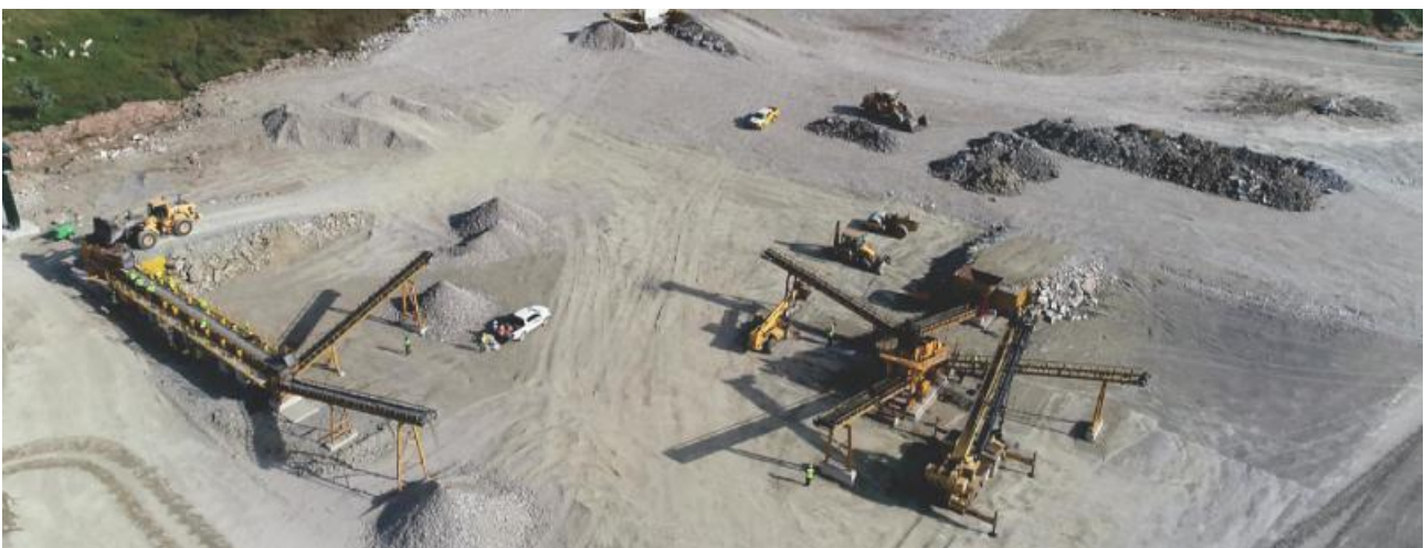
Figure 12. Commissioned Processing Plant
