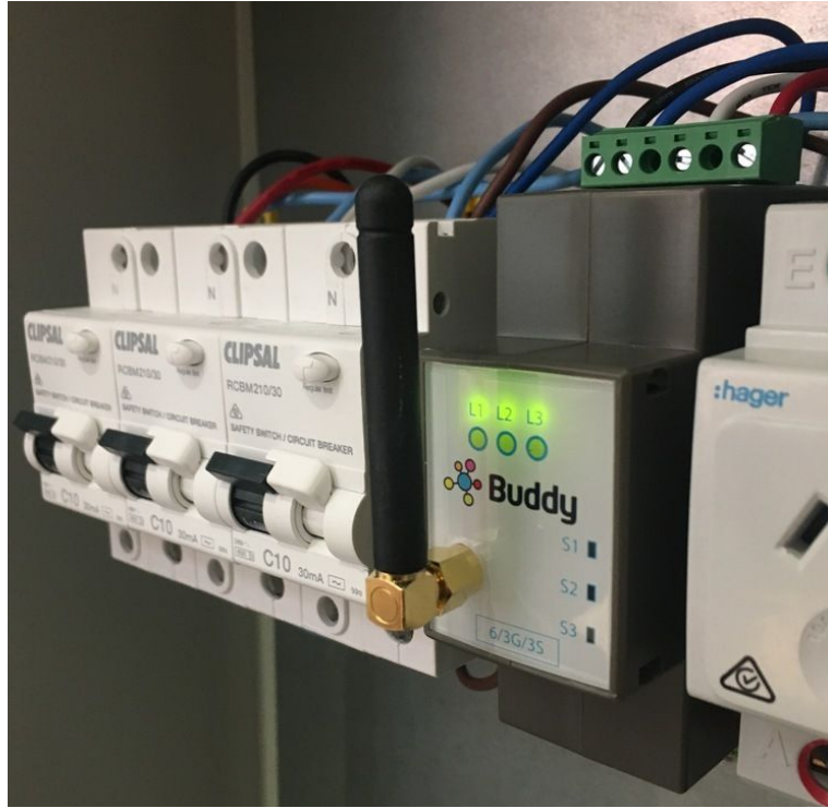
Figure 3 - WattWatchers device installed as part of a Buddy Ohm deployment.
