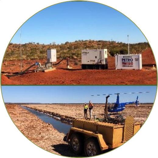
Brine Pumping from Bores and Trenches >260 Million litres successfully pumped to date
