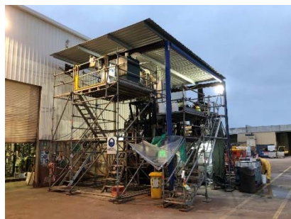
Acid Bake Pilot Plant
