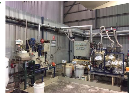
Phosphate Extraction Pilot Plant
