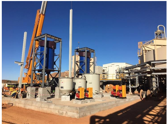
Figure 7: Regrind mill installation
