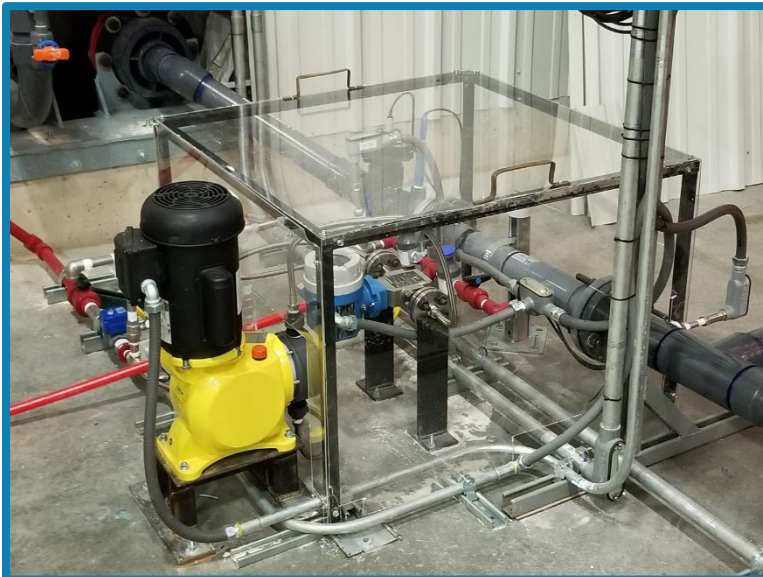
Sulfuric Acid Addition Pump
