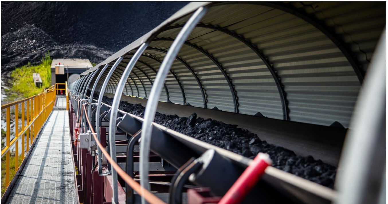
Figure 6: Raw coal conveyor feeding the Poplar Grove CHPP
