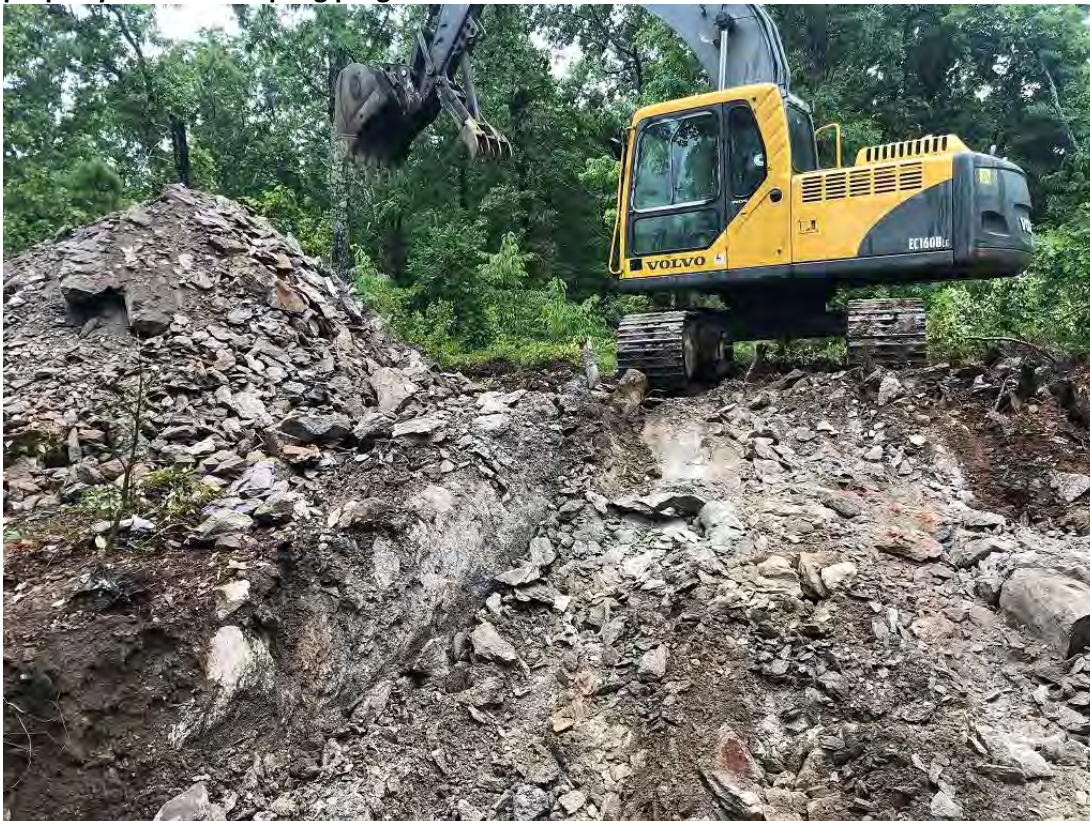
Figure 3: Excavation of 12 tonnes of weathered graphite rock from shallow pit (CMB001) at Ceylon property for bulk sampling program.
