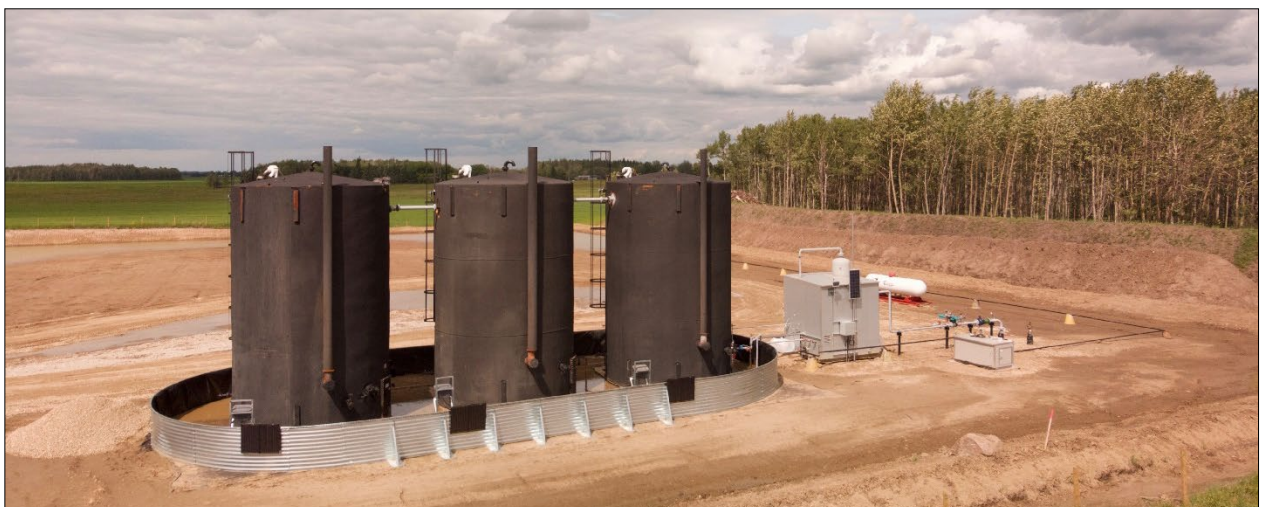
Figure 1 - Wizard Lake Surface Facilities
