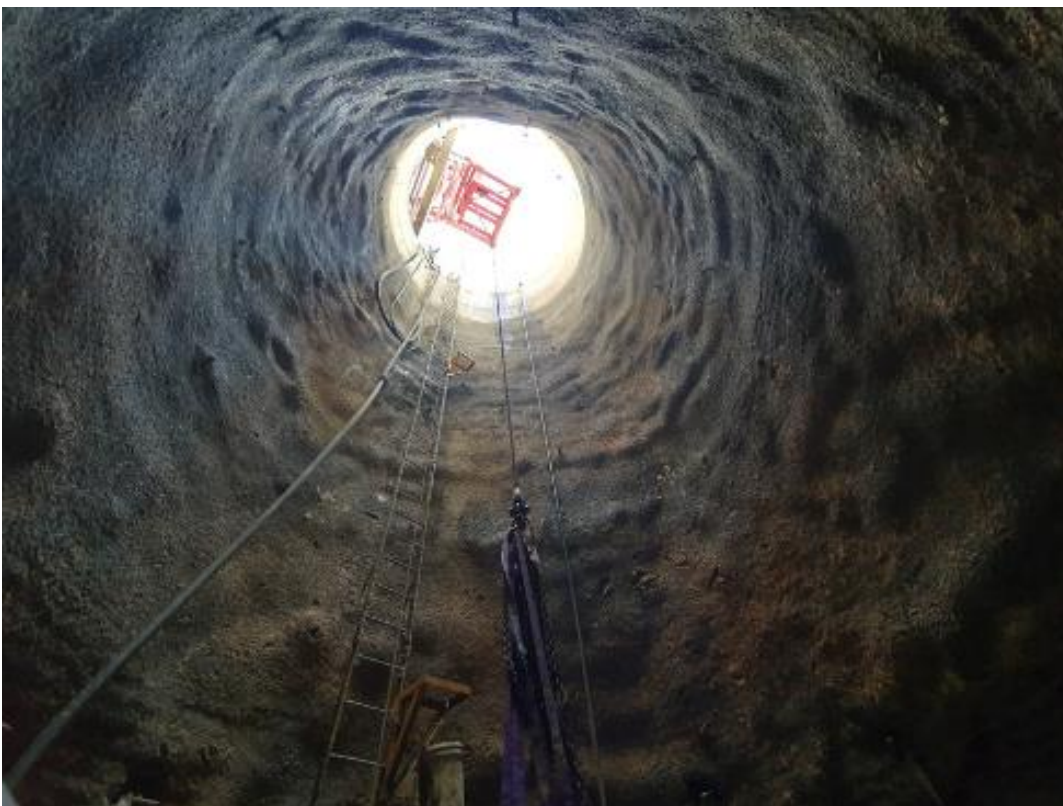
Figure 5 Woodlawn primary ventilation shaft.
