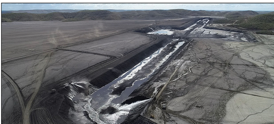
Figure 14: Hydraulic mining operations to date at the Century Zinc Mine
