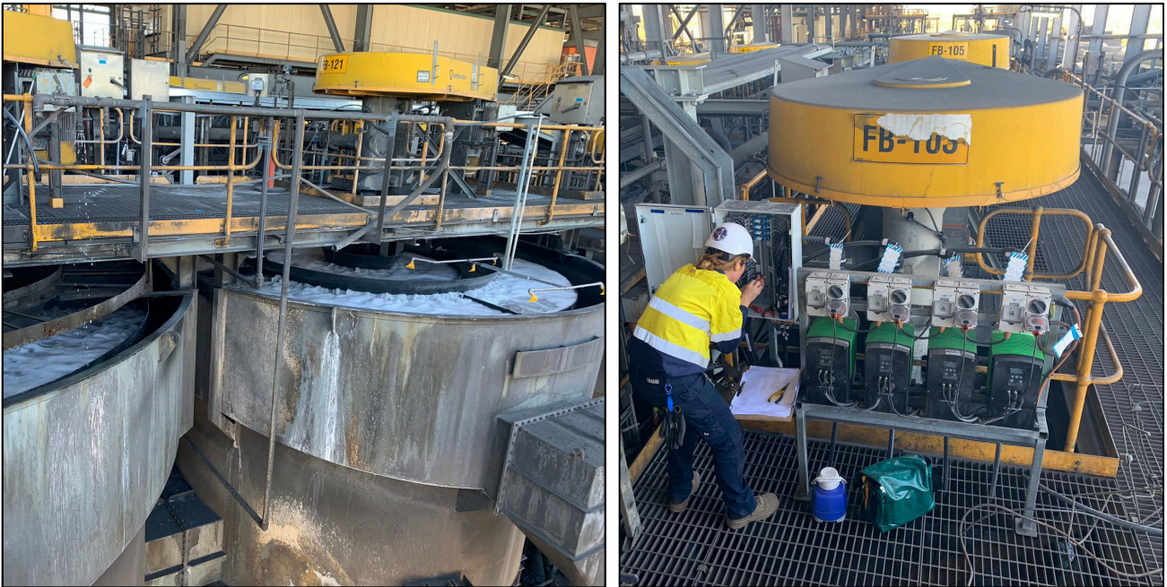
Figures 8 & 9: Water and air commissioning of cleaner 4B (left) & commissioning of new reagent dosing stations on cleaner 3B (right) in readiness for early August operations of the full cleaner circuit
