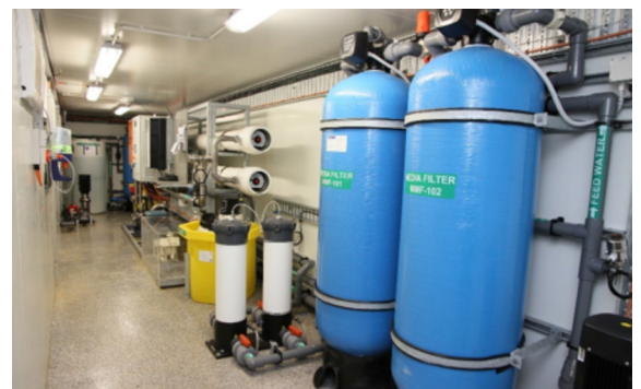
Figure 4 - Garden Island containerised desalination system
