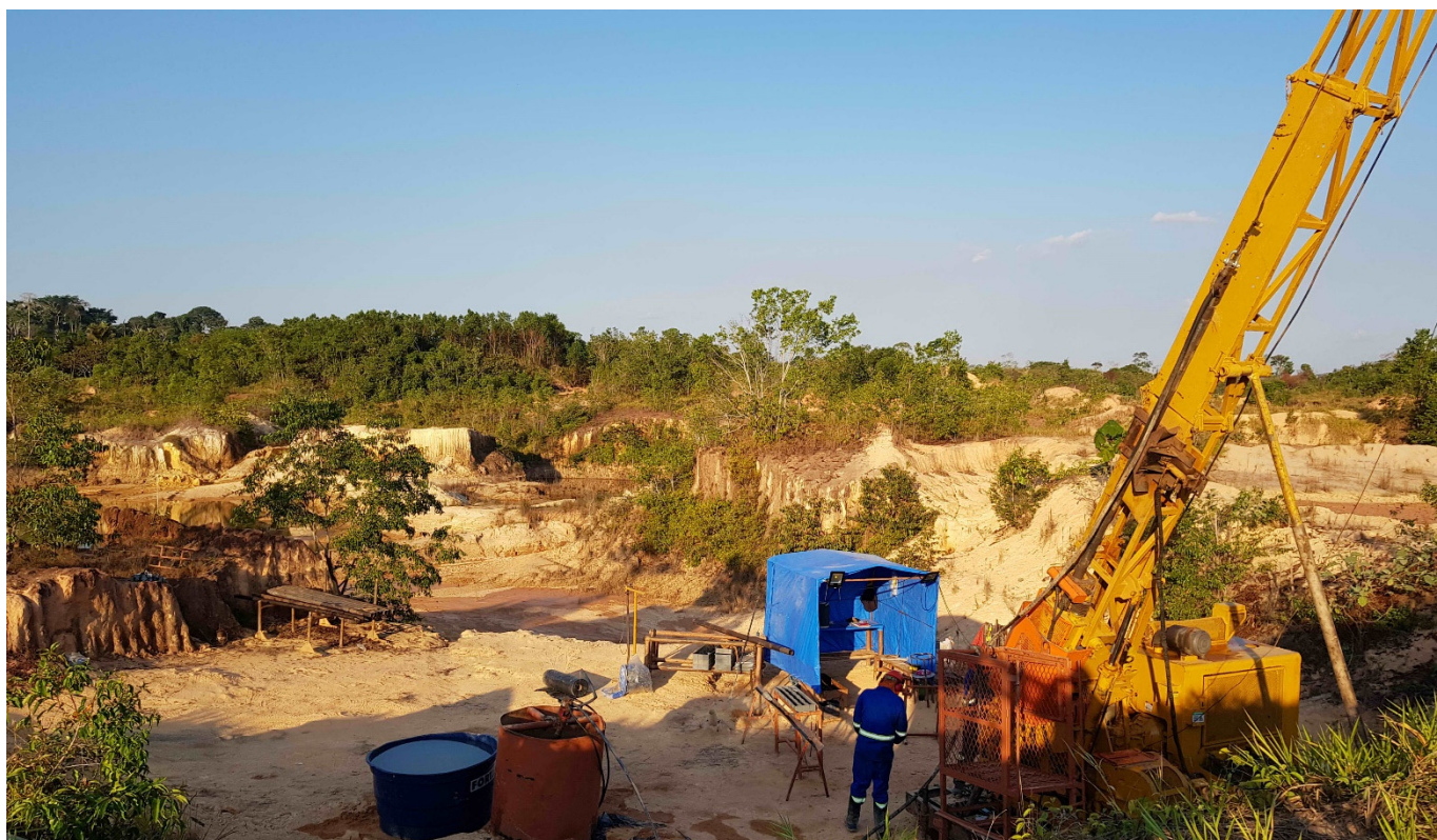
Figure 6: Drilling beneath the old workings at Dona Maria Prospect, Juruena Gold Project
