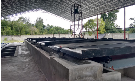
Figure 3(a): Shaking Table at the PTIM Plant
