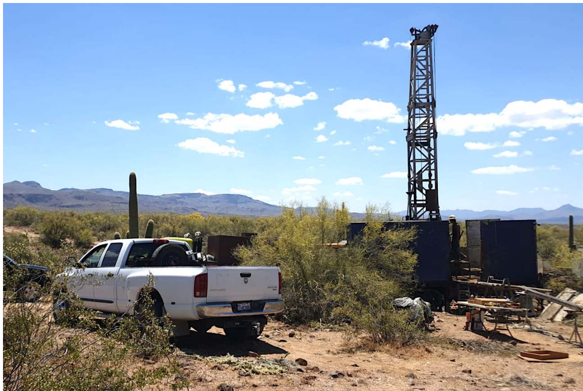
Figure 1: Diamond drill rig on site at the Big Sandy lithium project for the Company's 37 hole diamond drill program.
