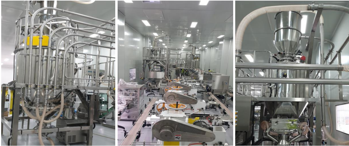
Installed plant and equipment for the new purpose-built Keytone Dairy manufacturing facility in New Zealand
