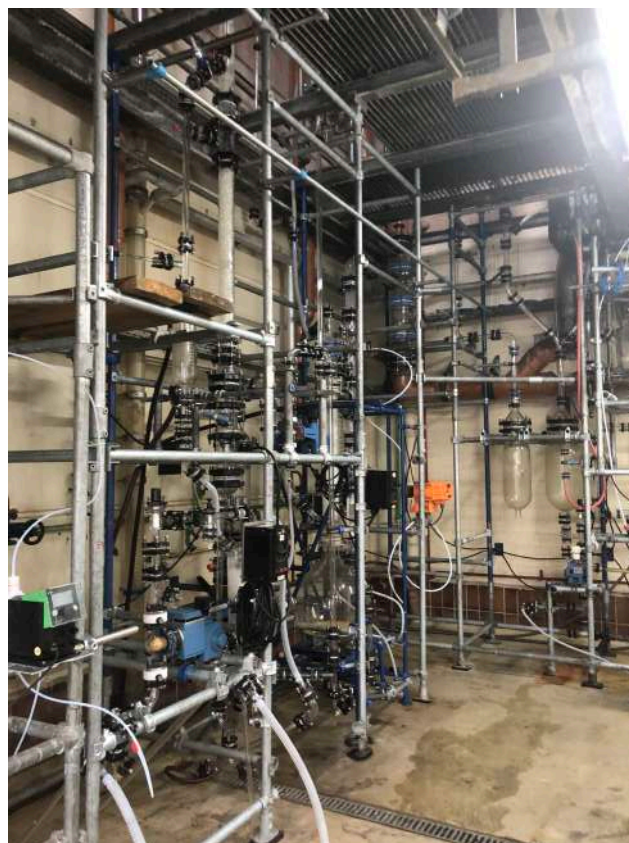
Figure 4: Bromine Pilot Plant Lower Floor
