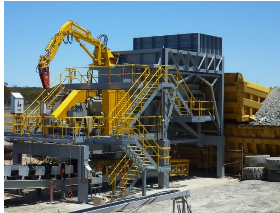
Kambalda Primary Crusher
