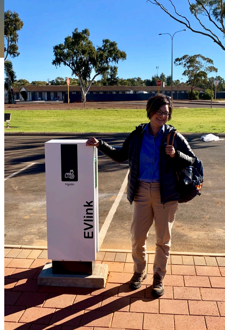
Ardea Chair, Katina Law, inspecting a recently installed EV charging station outside the City of Kalgoorlie Boulder Council office during a 2019 stake holder update meeting.
