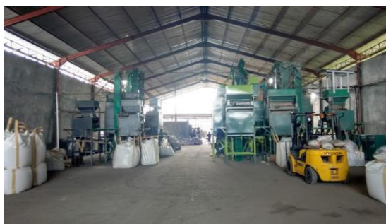
Figure 6-2 Electrostatic and electromagnetic separators installed at the Mandiri plant
