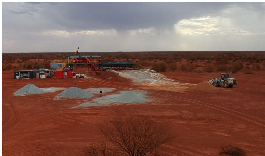
Concrete batching plant
