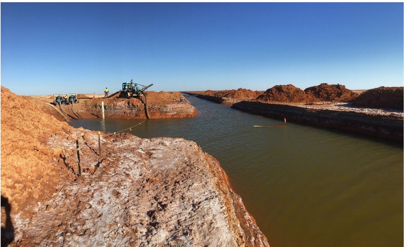
Figure 9: Brine Extraction Trench and Sump
