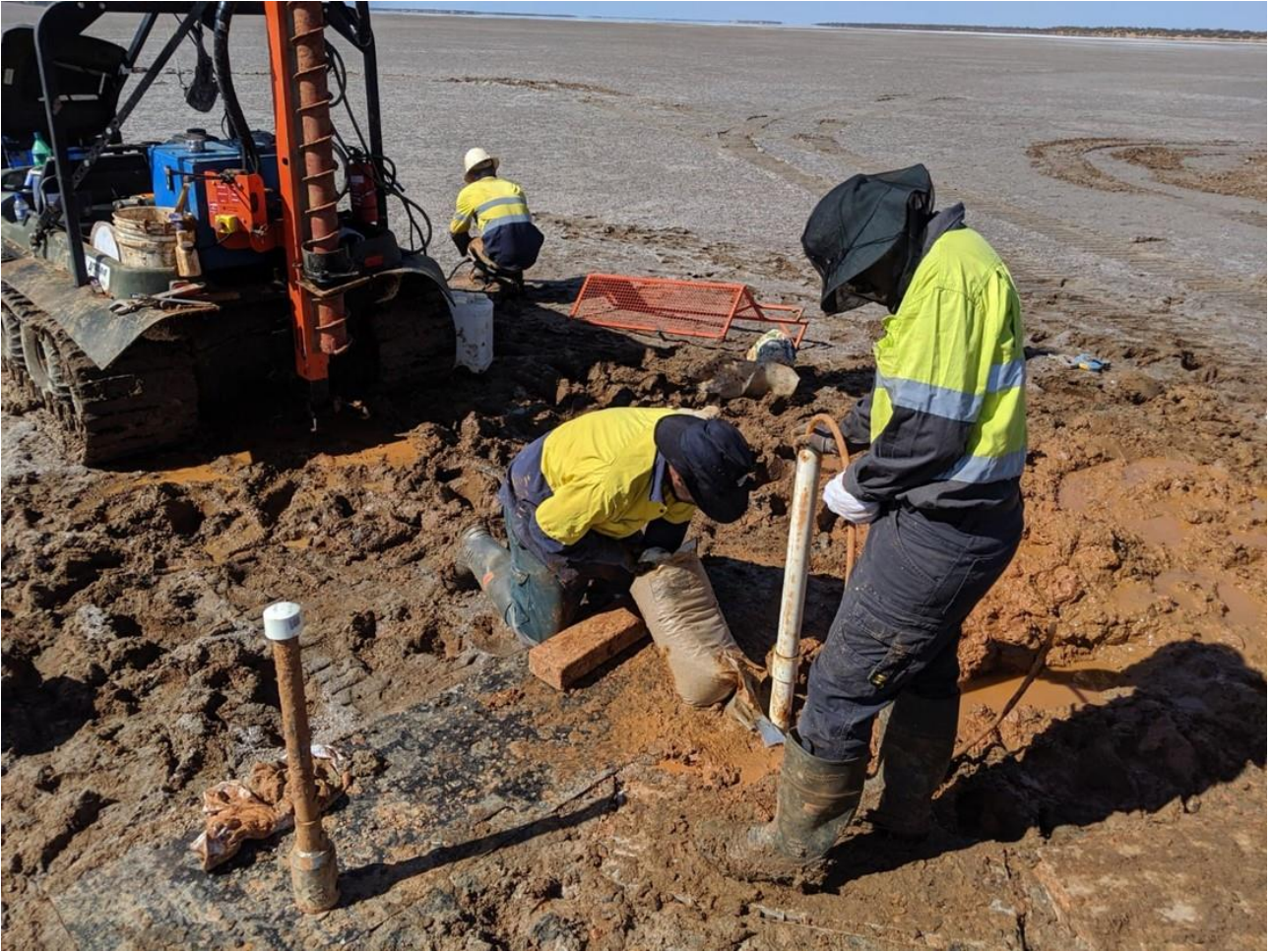
Figure 19: Installation of a monitoring piezometer after insitu geological and brine sampling at Lake Marmion
