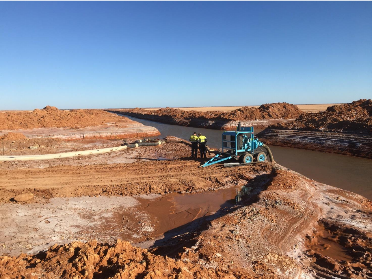
Figure 10: Pumping from the Brine Extraction Trenches
