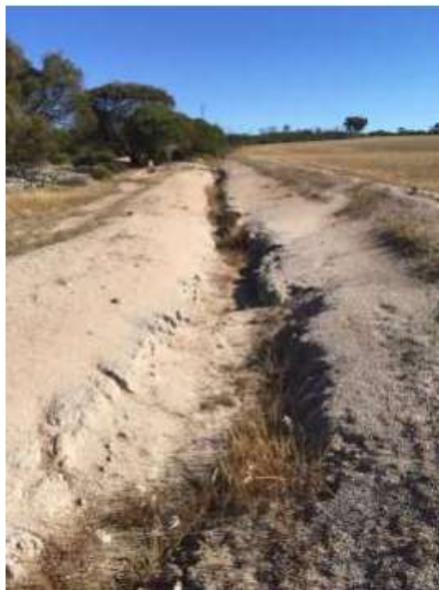
Figure 2: Erosional gully exposing outcropping kaolinic profile at surface
