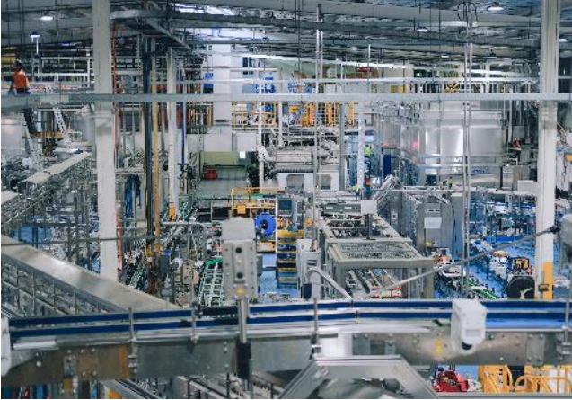
Overview of upgraded packaging line
