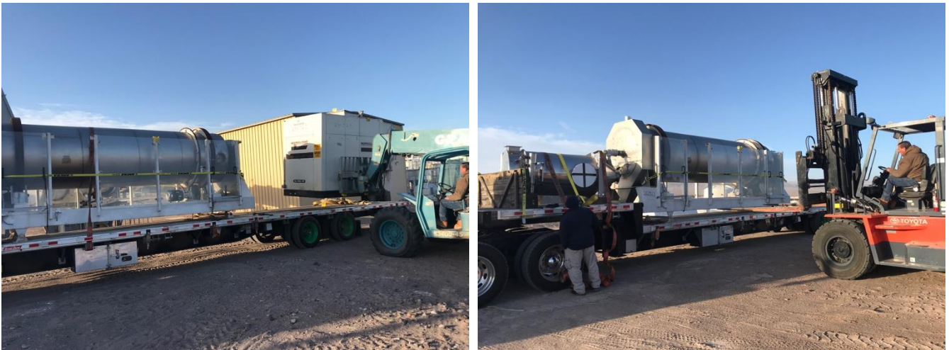
Figures 1 & 2 | Workers unloading boric acid production equipment at Fort Cady Borate Mine
