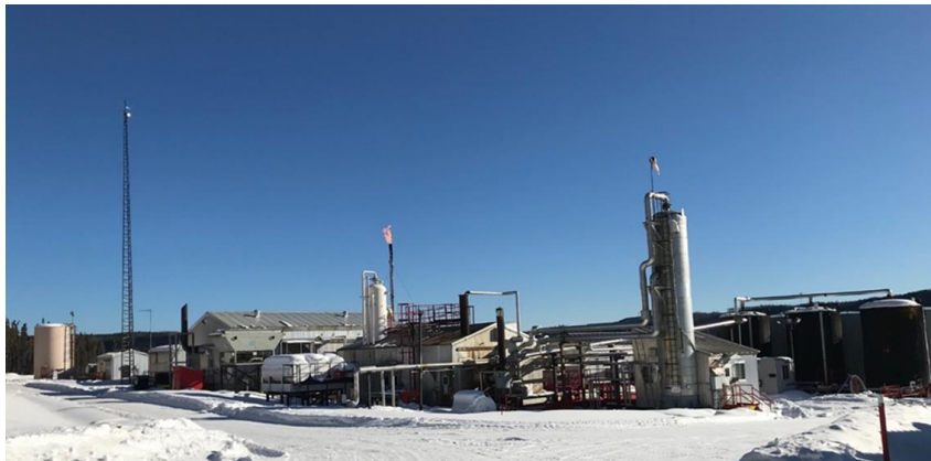
West 3 compressor and liquids handling
