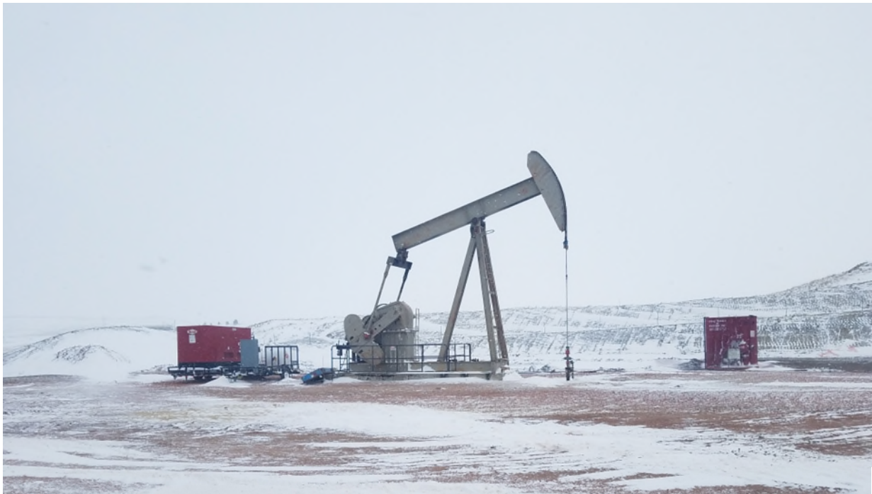
Pumping unit installed at Govt Kaehne #9-29 well.
