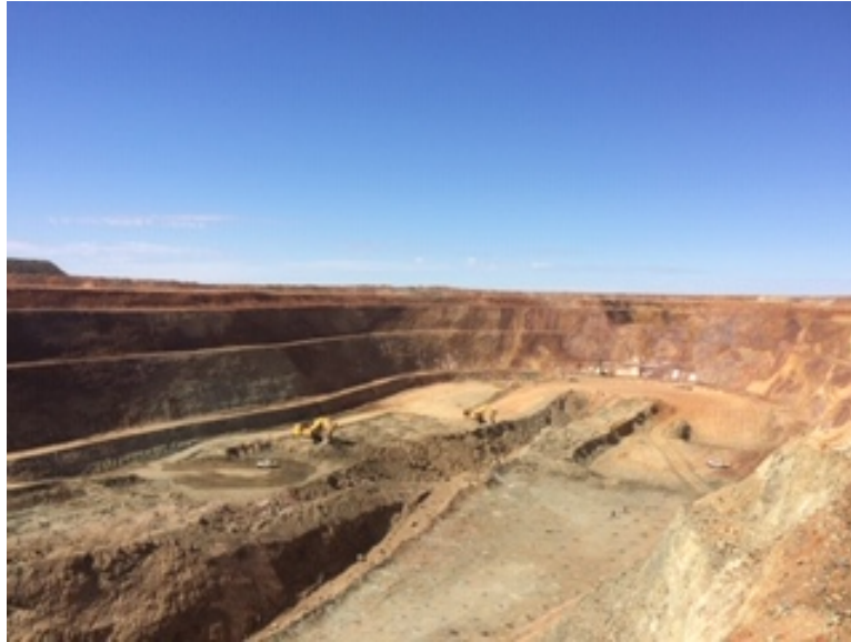
Photo 1: Cutback progressing on East and West side of Williamson open pit mine
