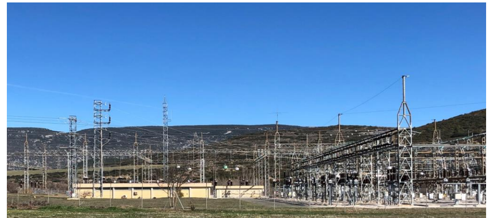
National Electricity Grid Substation in close proximity to mine site
