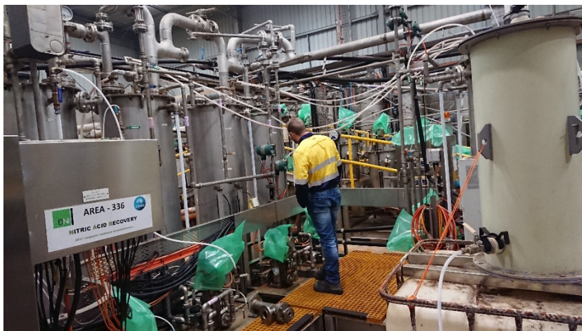
Figure 2: Examination of acid recovery section of the pilot plant
