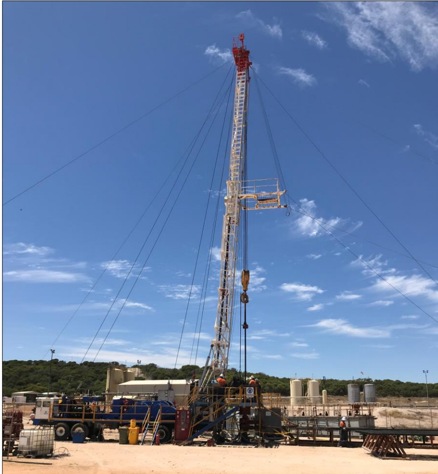
Refine Rig #1 currently in the Perth Basin and will shortly be mobilised to Key's Mount Horner site.
