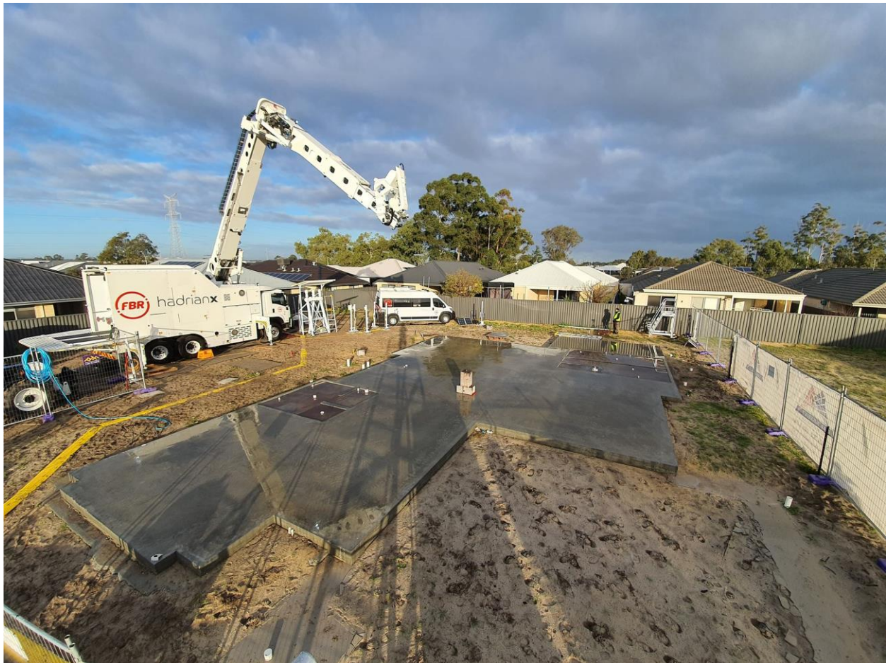
The Hadrian X® preparing to build its first display home in a residential development
