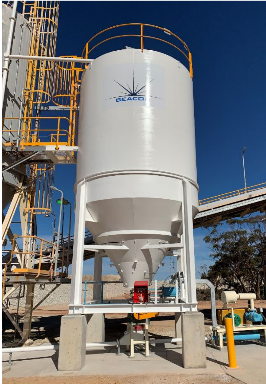
Figure 1: Jaurdi Gold Project – Additional Lime Silo
