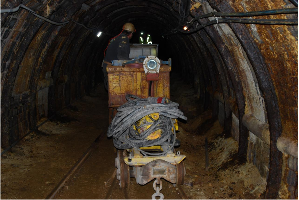
Image 2: Drill rig and ancillary equipment being mobilised to the underground Andrej adit
