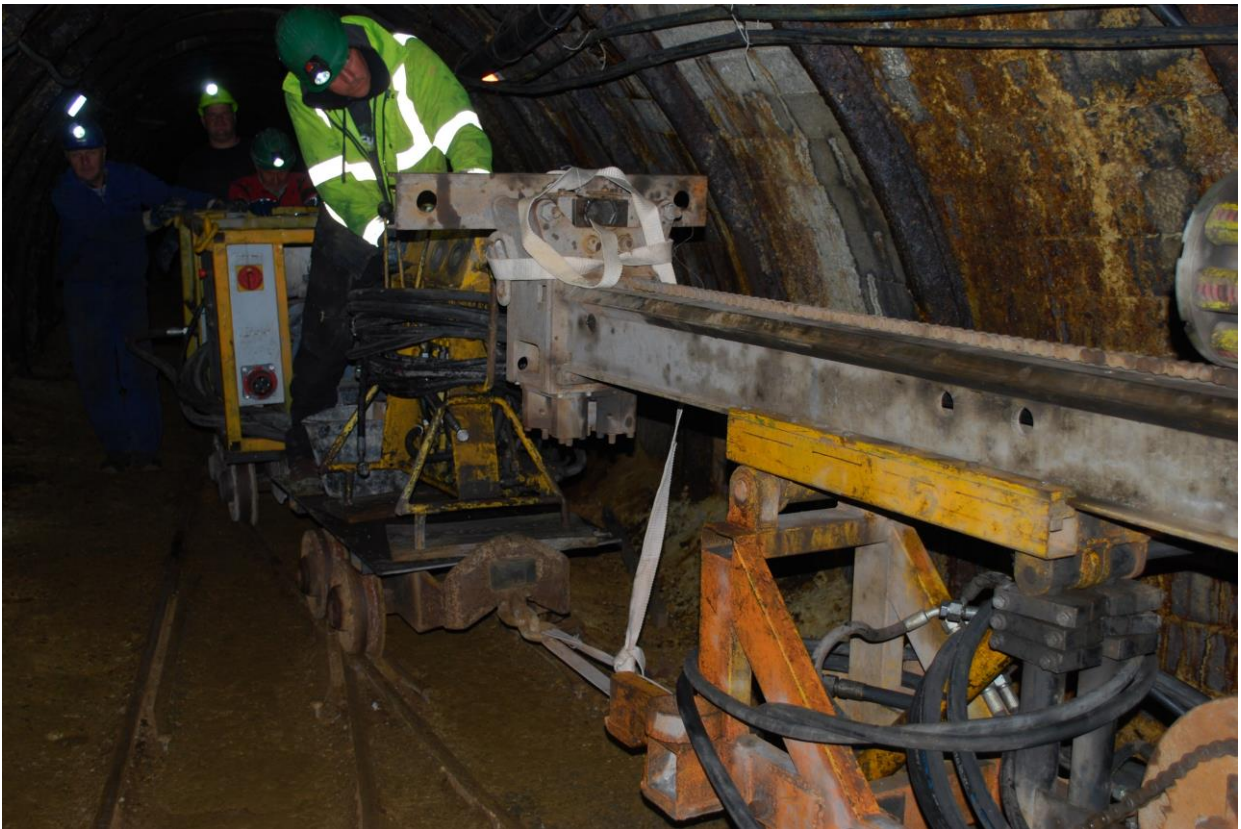
Image 3: Drill rig and ancillary equipment being mobilised to the underground Andrej adit
