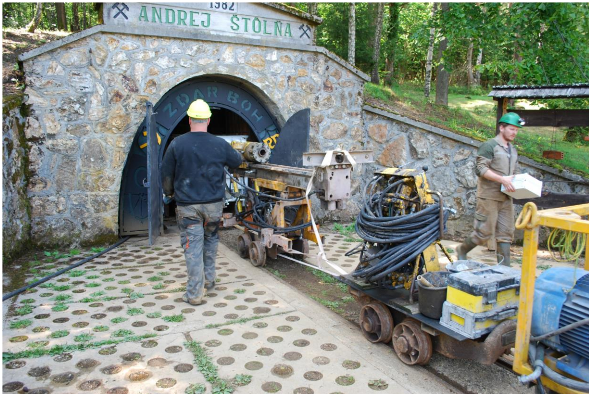
Image 1: Drill rig and ancillary equipment at the entry to the underground Andrej adit
