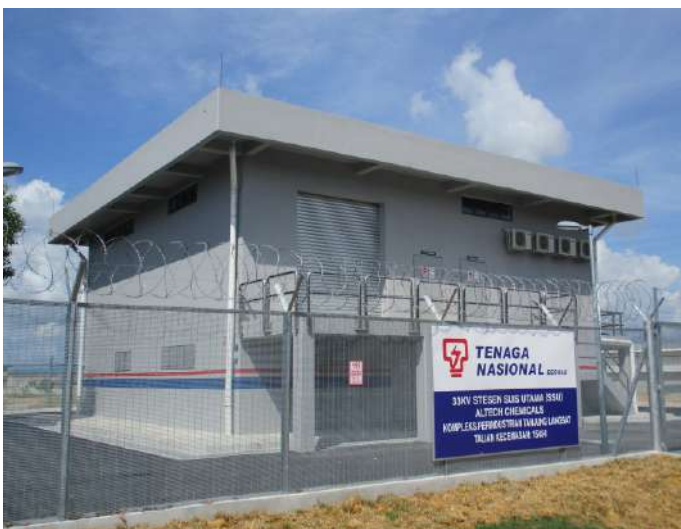
Completed electrical substation, Altech HPA plant site
