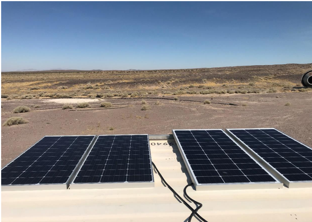
Figure 2 | Photo showing solar PV modules on the Company's site office
