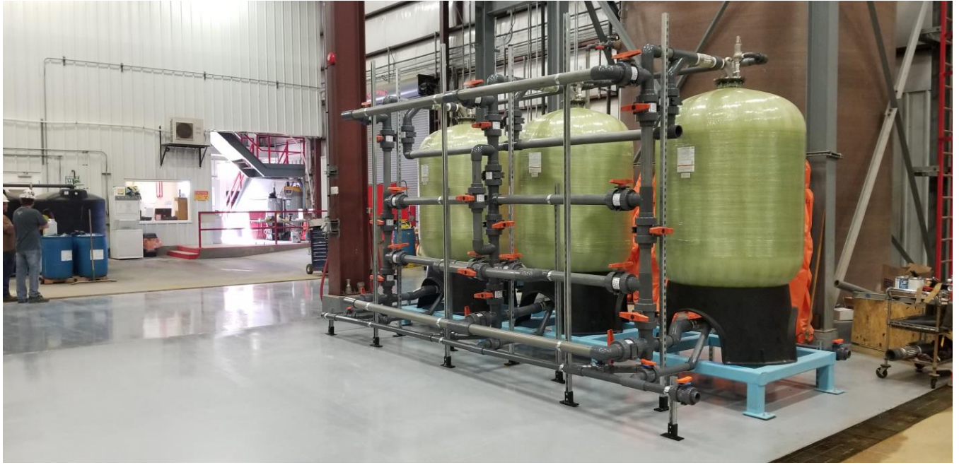
Figure 5: Constructed Ion Exchange Test Columns for MU1A Field Demonstration
