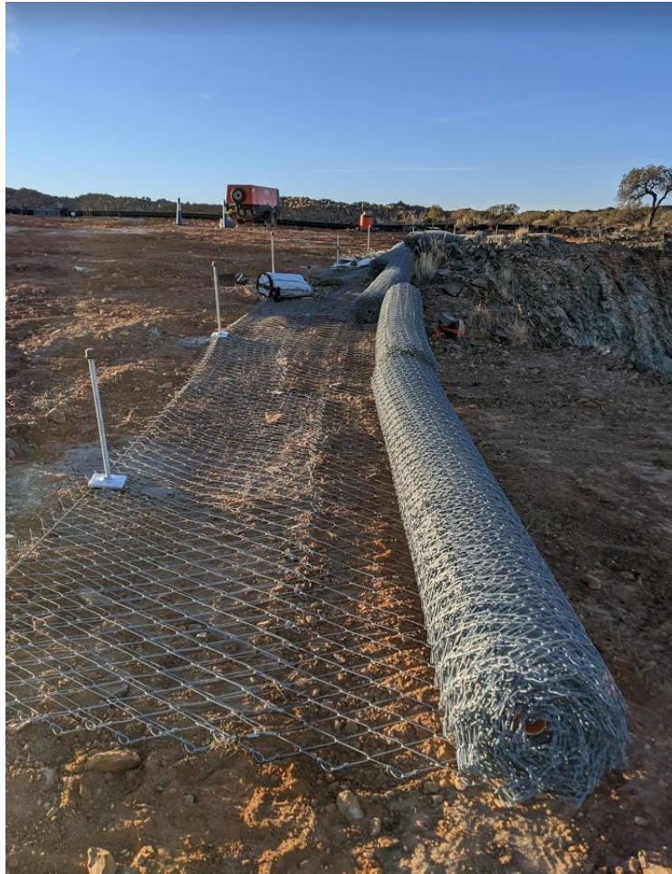
Image 3: Ground support being anchored above the portal in preparation for securing to the Paris Pit wall face above and around the new portal
